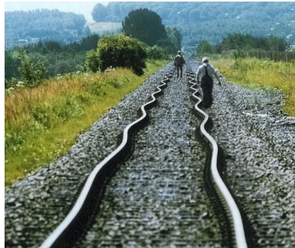
Fig. 1 Track shift after a test run with an older diesel engine (from [Köhler et al., 2003])
